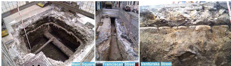
Fig. 6 Examples of repair works of paving realized by layering impermeable materials such as concrete. Source: B. Resutík
